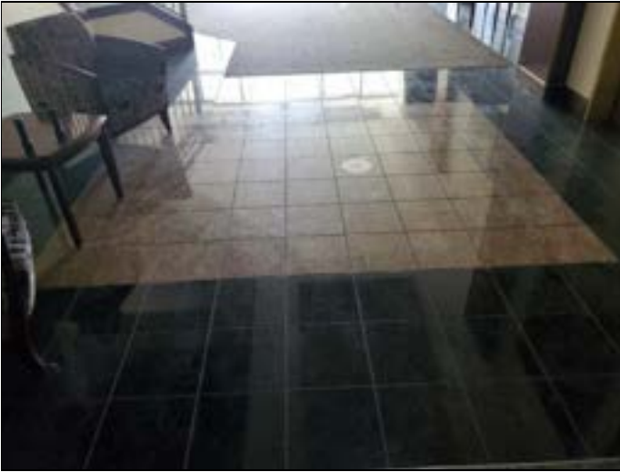
31. Assumed ACM: Grout and mortar associated with 12"x12" black and beige stone tiles, first floor
