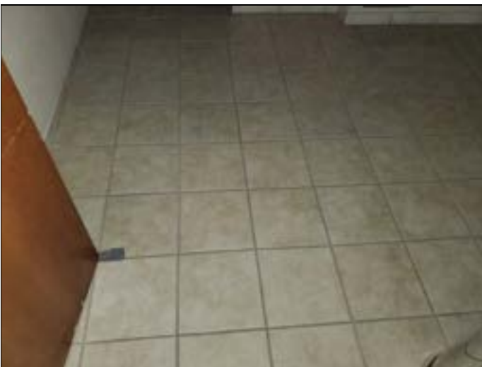
35. Assumed ACM: Grout & mortar to 12"x12" beige and cream ceramic tiles, restroom floor, 2 nd floor
