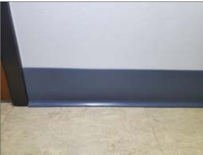
15. Samples 09A-09C: 4" grey cove base with white mastic, second floor
