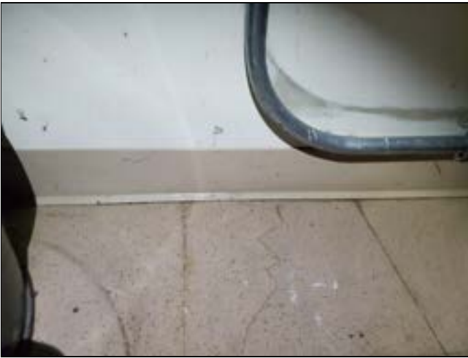
25. Samples 19A-19C: 4" tan cove base with tan mastic, first floor
