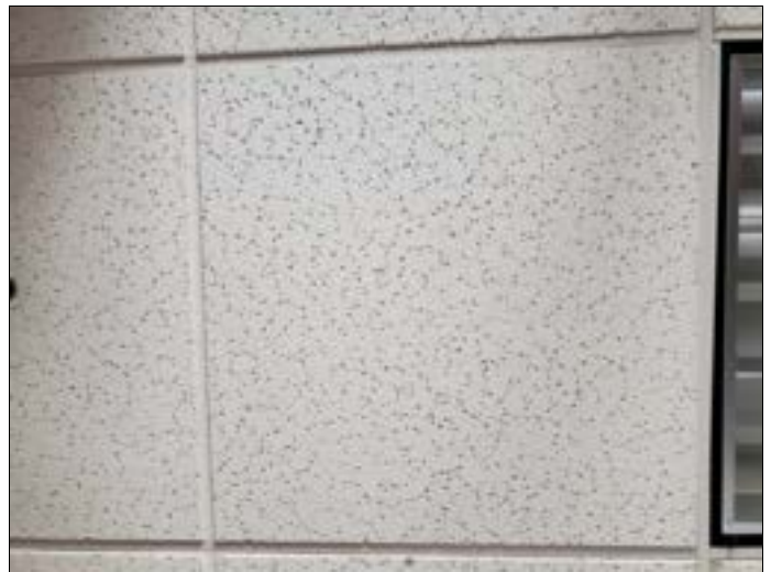
10. Samples 04A-04C: 2'x4' ceiling tile with pinhole and fissure pattern, second floor
