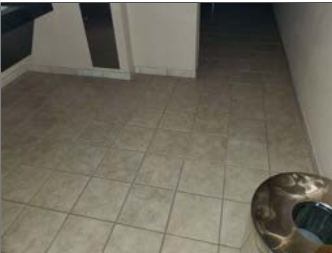
33. Assumed ACM: Grout & mortar to 12"x12" beige and cream ceramic tiles, restroom floor, first floor
