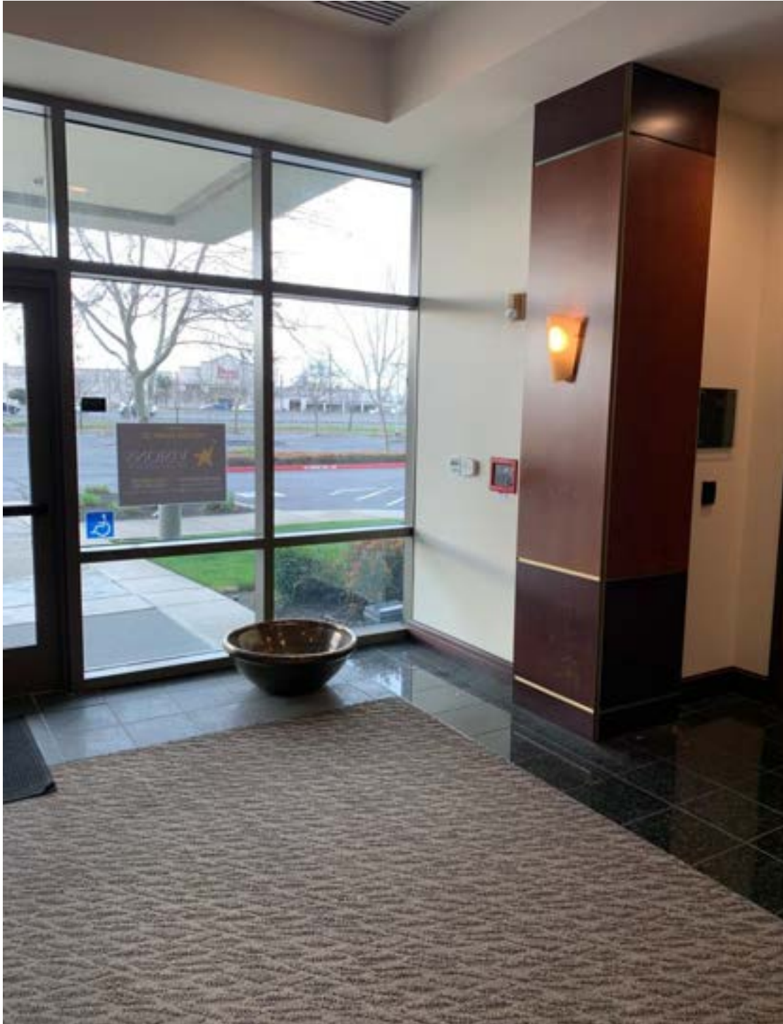
Addendum No. 1 – Attachment 1.12 Visions In Education – Tenant Improvement Project #24-01 Fire Alarm Panel
