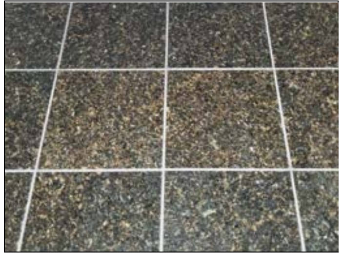
32. Assumed ACM: Grout and mortar associated with 12"x12" black and beige stone tiles, second floor
